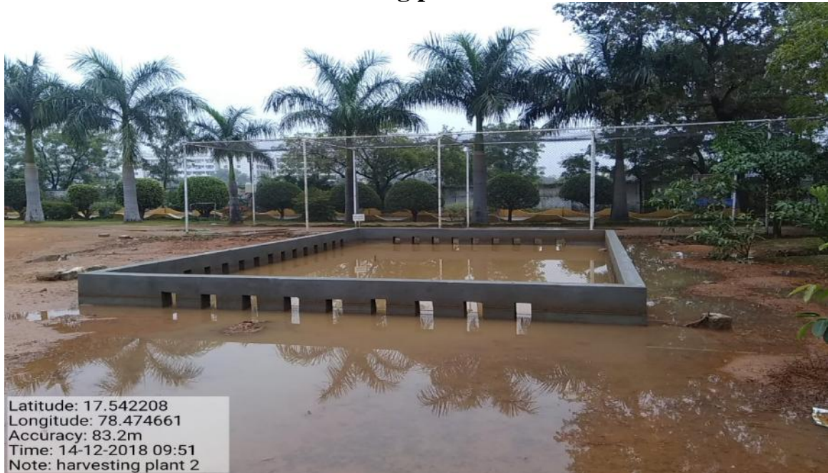
Fig 1(a): Surface Runoff Water harvesting plant in College Playground (front view)
