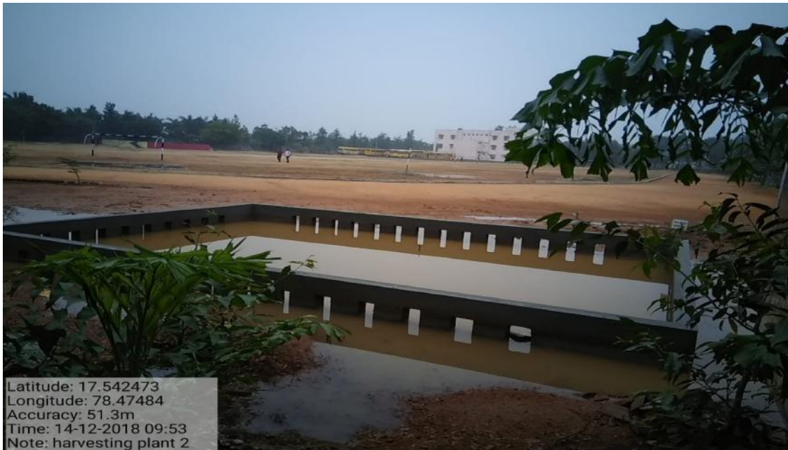
Fig 1(a): Surface Runoff Water harvesting plant in College Playground (side view)
