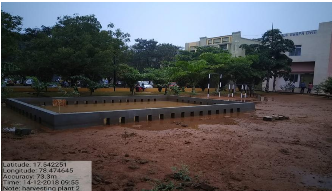
Fig 1(b): Surface Runoff Water harvesting plant in College Playground (left view)
