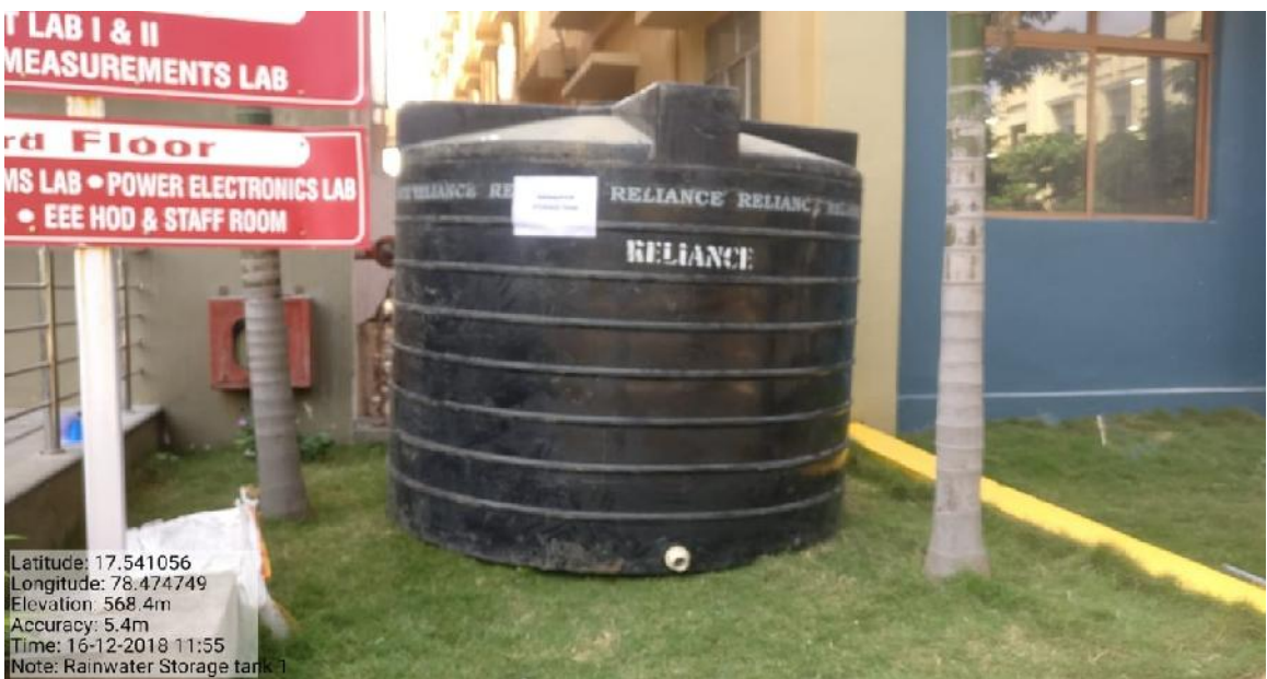
Fig 2: Rooftop rain water storage tanks Capacity each 5000 liters
